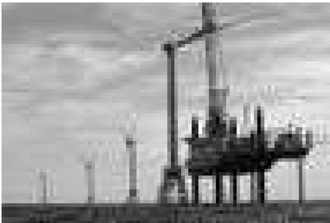
Block Island, R.I.: Deepwater Wind installing the first offshore wind farm at Block Island, Rhode ... [+] NEWSDAY VIA GETTY IMAGES
